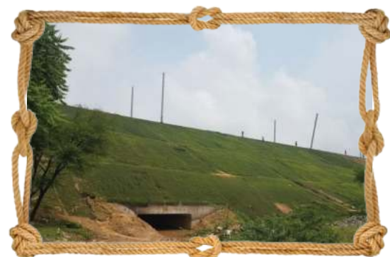
Figure 2. Erosion control measures using coir geotextile on railway embankment, Pali, Rajasthan (a) before construction (b) after construction
